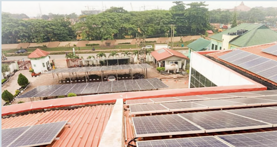
Figure 6 Havenhill’s solar panel installation
