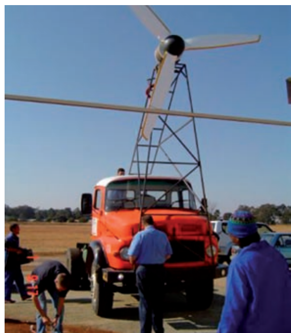
Kestrel Wind Turbines in South Africa supported by GroFin.
